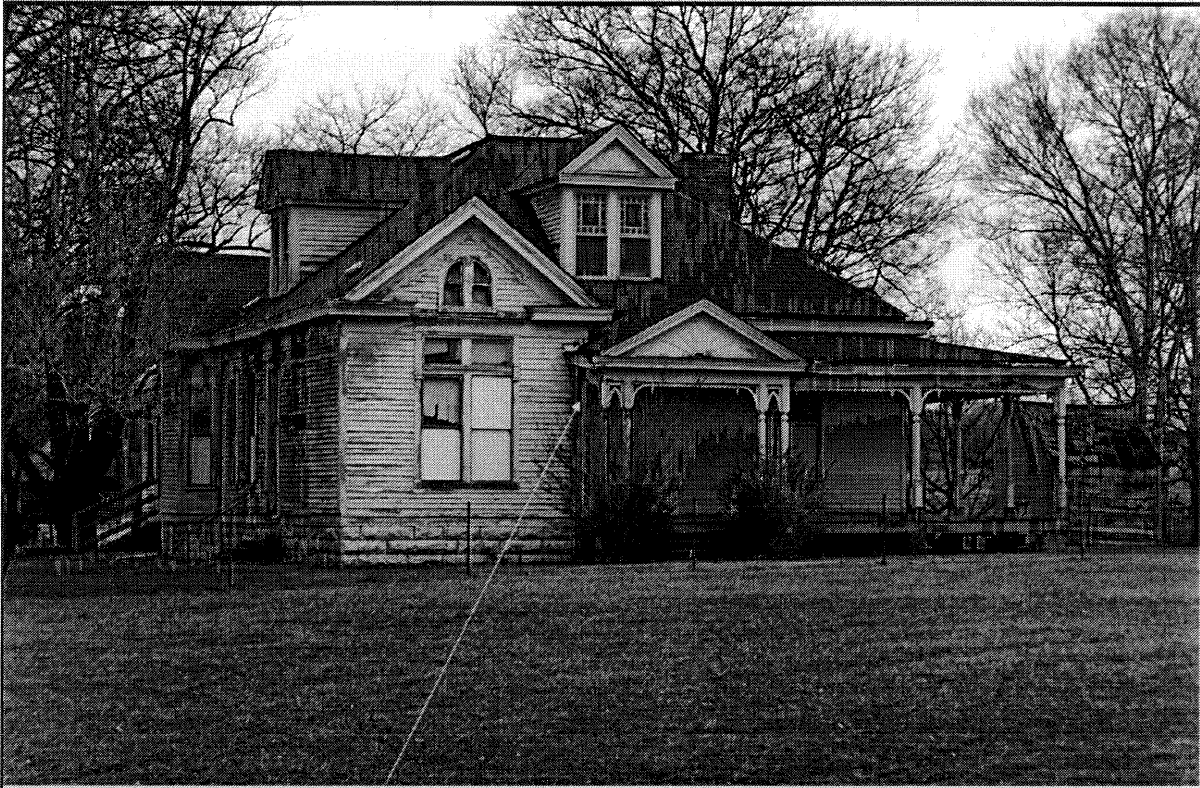
Front porch has settled and a lot of the trim has separated. This has allowed weather to cause dry rot of gutter boards, framing and soffits. This separation from settling has happened all the way around the home.
