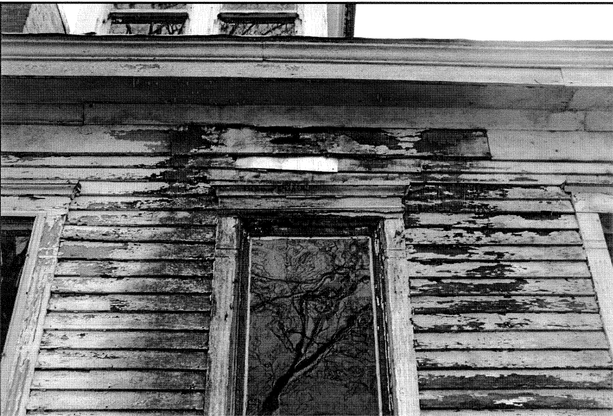
Most of the outside and inside damage was caused from the gutter system leakage over years
