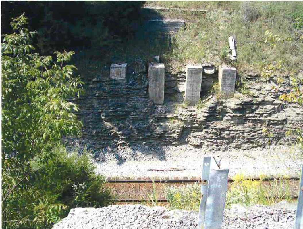
8) Old Bridge west abutment foundations at CSXT Railroad from Wilson Pike near STA 610+00
