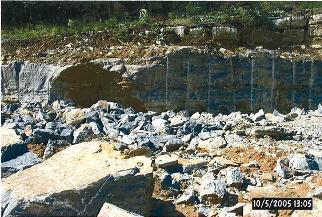
3) Pre-split rock cut near STA 463+00. Note the stained rock with a small solution cavity in the middle to left of center.
