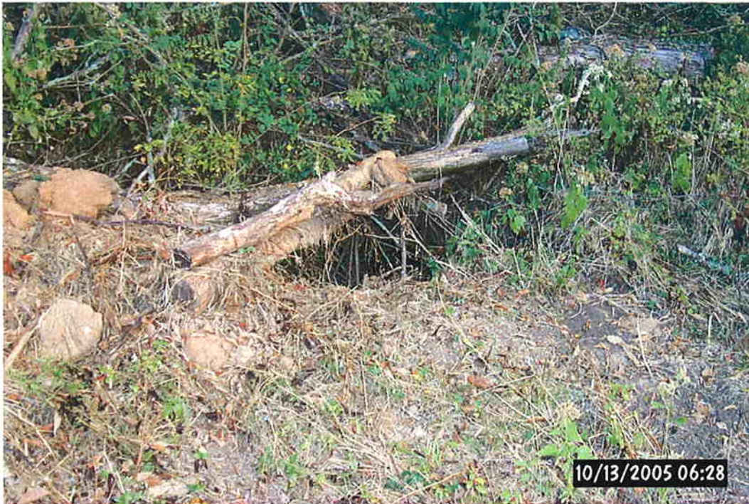
1) Suspected Sinkhole near STA 434+40, 20-ft right
