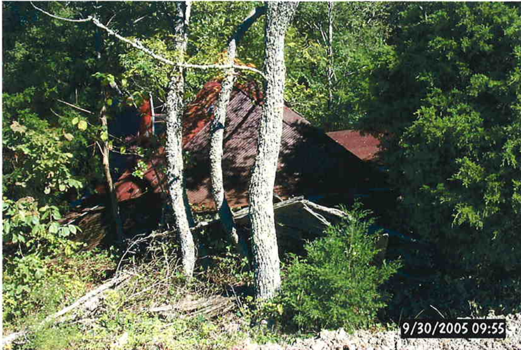
5) Ruin of shed near STA 469+00
