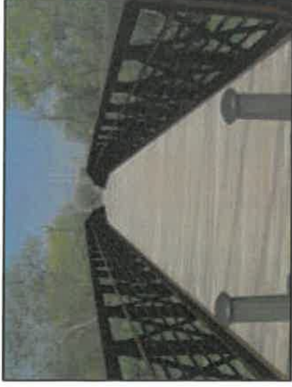
This existing pedestrian bridge linking the Fort Granger site with the historic train depot parking lot is a good model for additional future bridges.
