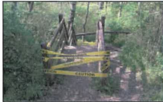
Access to the fort from Pinkerton Park includes facilities in serious need of repair.
