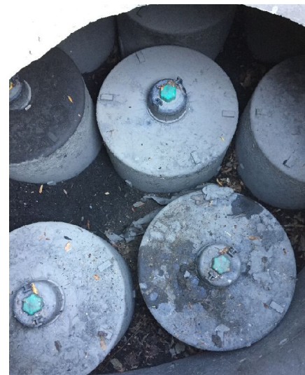
Figure 8: Water quality unit
