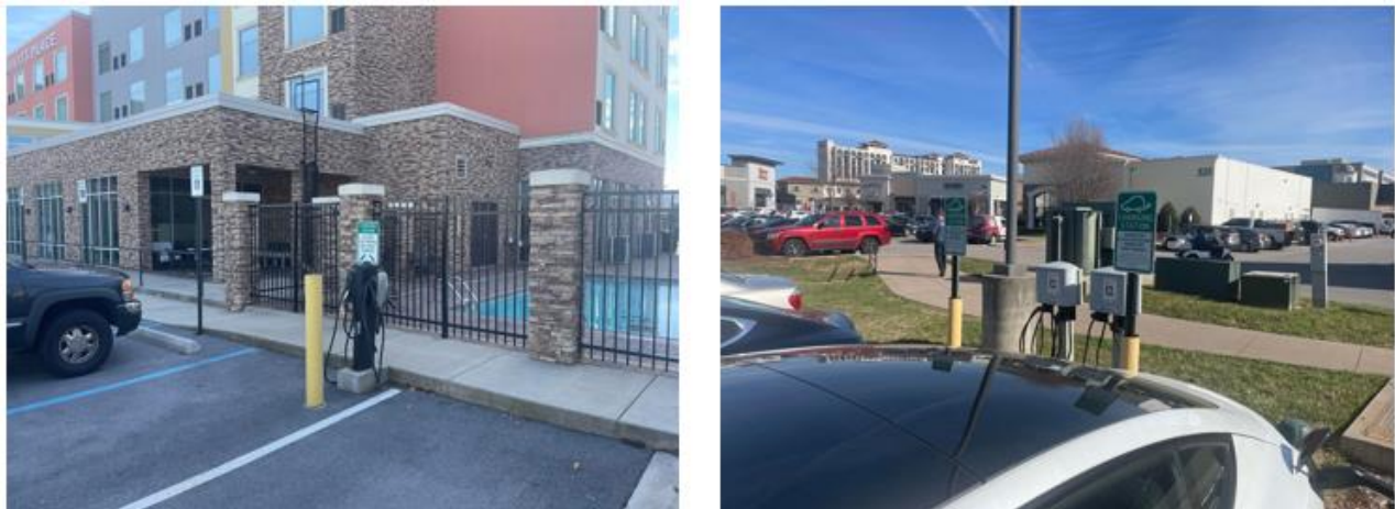
Figure 1. Electric vehicle charging stations at a hotel and at a shopping mall (private). Source: ITE.
