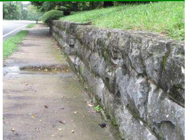
The stone retaining wall in the 100 block of Lewisburg Avenue is a historic feature of the neighborhood.
