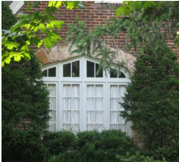
The arched opening and multiple-pane window at 920 Fair Street is an important component of the dwelling's Tudor Revival style and character.
