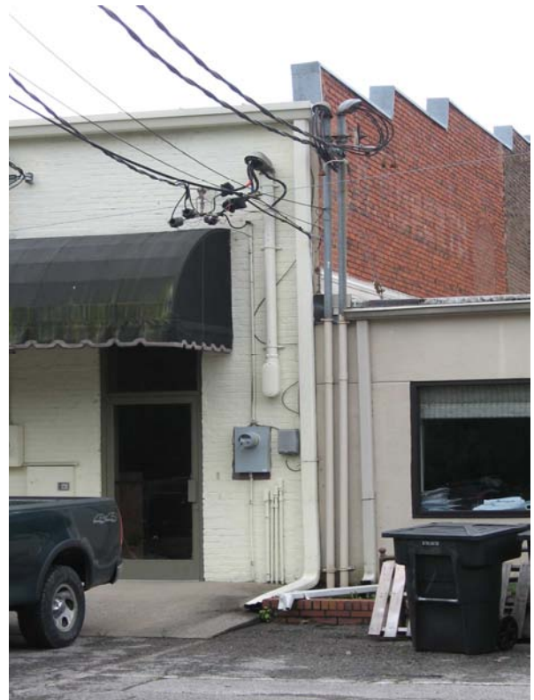
The building at 338 Main Street has appropriately placed meters and equipment on the rear elevation.
