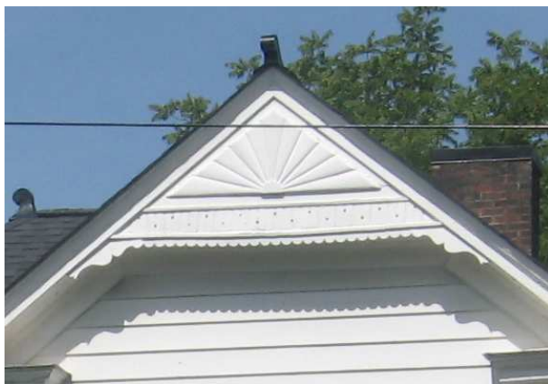
The paint on this historic vergeboard at 1324 Adams Street maintains historic character and helps with physical preservation.
