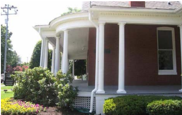
The downspout on 143 Fourth Avenue North uses placement at a corner and coloring that matches its adjoining surface to minimize its visual effect.
