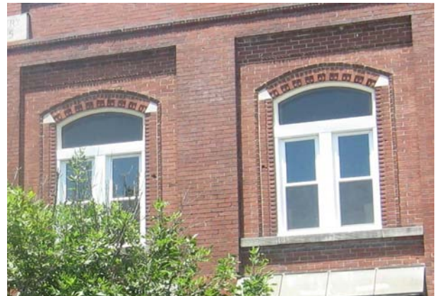
The inset openings, corbelled brickwork, and concrete sills of the windows at 428 Main Street should be preserved and remain visible.
