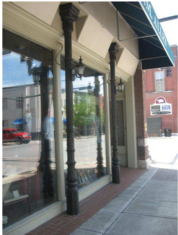
The painted finish of these cast iron columns at 347 Main Street helps to protect them.
