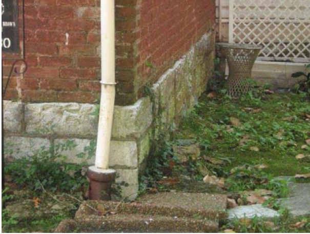
Above ground foundations defined by an alternate material from the exterior walls, such as this one at 724 Fair Street, were common on historic buildings.
