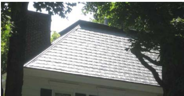
The metal roofing materials at 1327 Adams Street contribute to the house's historic character.
