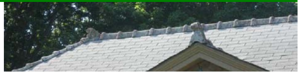
Retaining elements like the crestring and end ridge caps on 906 Fair Street helps to preserve historic character.
