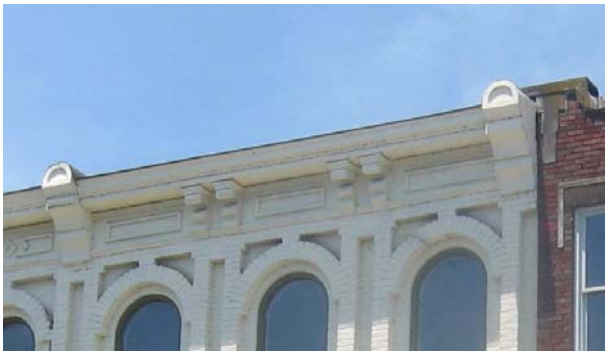
Metal cornices like the one on 334 Main Street were often used on commercial buildings from the late 1800s.
