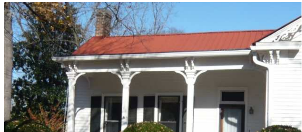
Careful selection of the 5 V metal used on this Fourth Avenue South home enabled the roof to retain its historic appearance.
