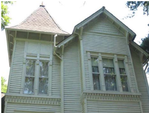
The decorative siding on the house at 819 West Main Street contributes to its Queen Anne character.
