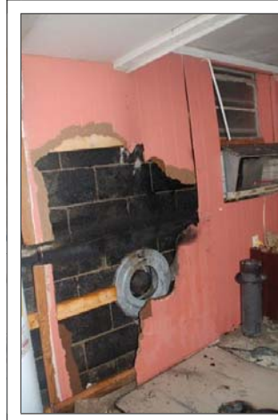
Basement where a fire started in the home at 213 Ash Dr.
