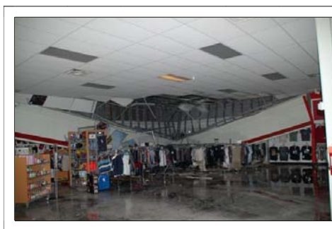
TJ Maxx ceiling partial ceiling collapse.
