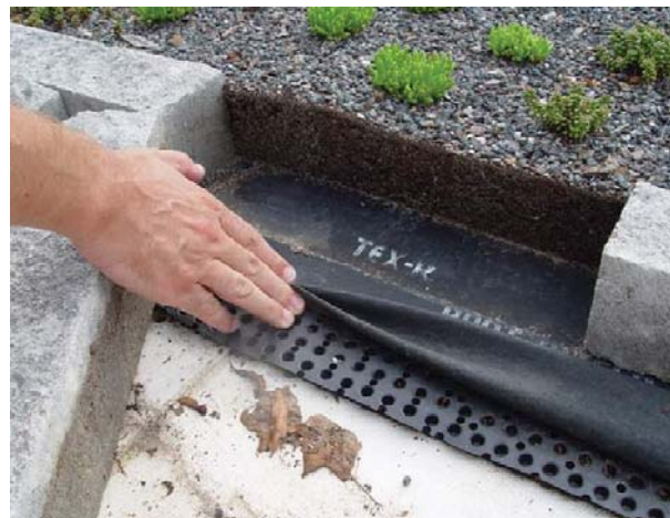
Figure 9.1. Photos of Vegetated Roof Cross-Sections (source: B. Hunt, NCSU)
