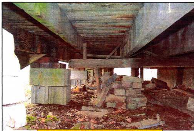
Entire wrap around porch is poorly supported.
