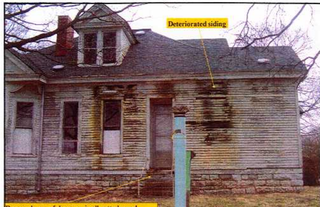
Deteriorated siding Recessed area of doorway is all rotted wood. Approx. a 3'x3' landing.
