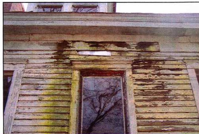
Most of the outside and inside damage was caused from the gutter system leakage over years
