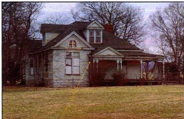
Front porch has settled and a lot of the trim has separated. This has allowed weather to cause dry rot of gutter boards, framing and soffits. This separation from settling has happened all the way around the home.
