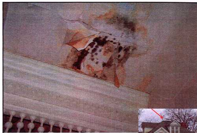
Center of house- Caused by Widow's Peak leaking
