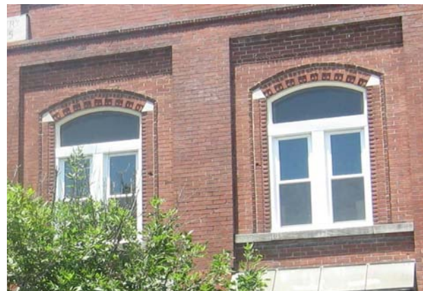
The inset openings, corbelled brickwork, and concrete sills of the windows at 428 Main Street should be preserved and remain visible.
