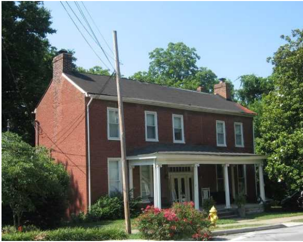
The chimneys at 724 Fair Street contribute to the balance so important to the house's Federal style.
