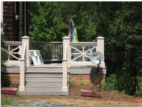
Satellite dishes should be mounted at rear elevations where they are not readily visible from the street.
