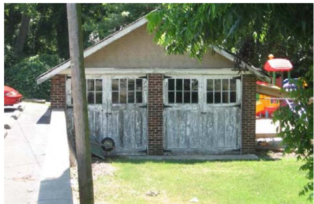
Remaining original doors like these on 137 Fourth Avenue North should be retained and may be retrofitted to accommodate modern conveniences.
