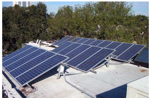
Solar panels are encouraged; they should be placed out of view from the street.
