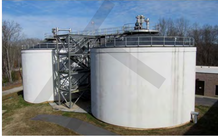
Figure 2 Anaerobic Digesters at Gilder Creek WWTP, Greenville, SC
