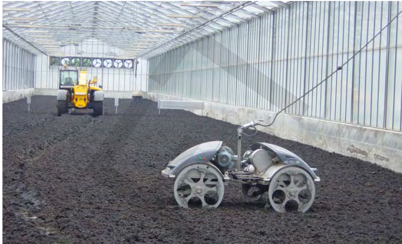
Figure 4 Parkson Thermo-System Solar Dryer in Okeechobee, FL
