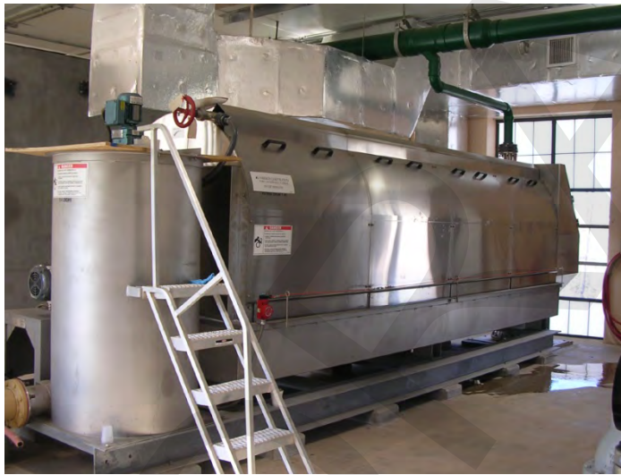
Figure 1 RDT with Enclosure at Gilder Creek WWTP, Greenville, SC
