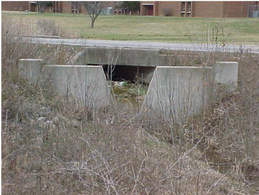
Figure 4 – V-notch outlet structures are recommended because they offer a wide range of control for large, medium, and small storms, and they are used in this example.
